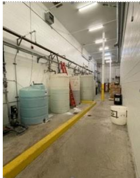
Figure 2 - Jordan River Service Center Mechanical Room
