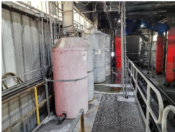
(Figure 1- Warm Springs Vehicle Wash Soap Tank)
