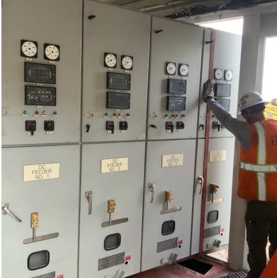
Old DC Breakers
