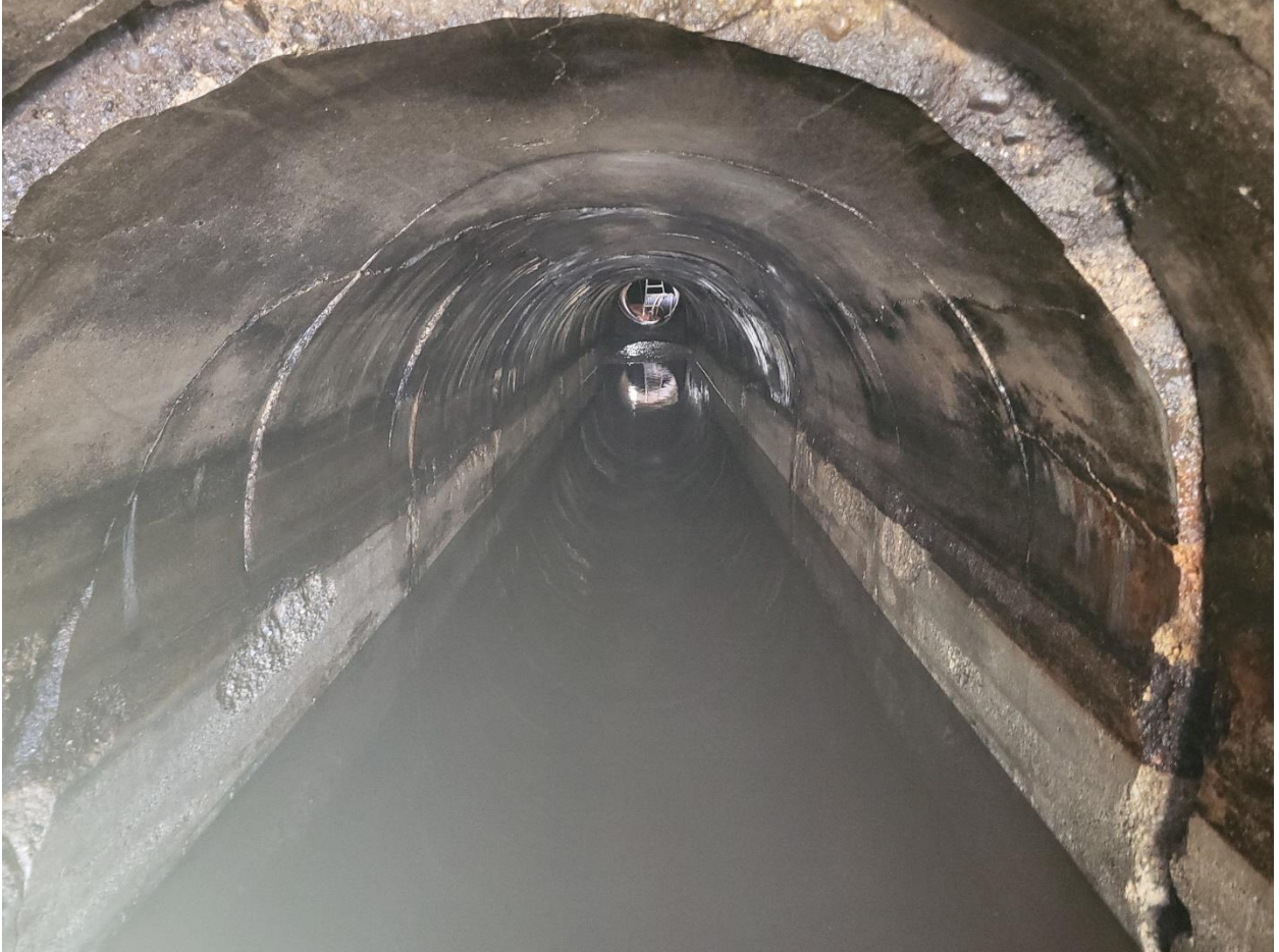
Image 1: Cracked and settled
