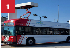
Meadowbrook Bus Charging Infrastructure
