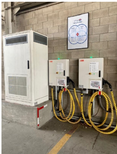
Plug-in charging infrastructure
