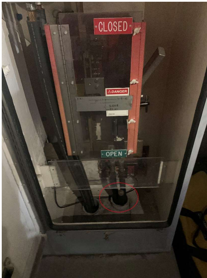
Cut POS feeder cable inside DS-08
