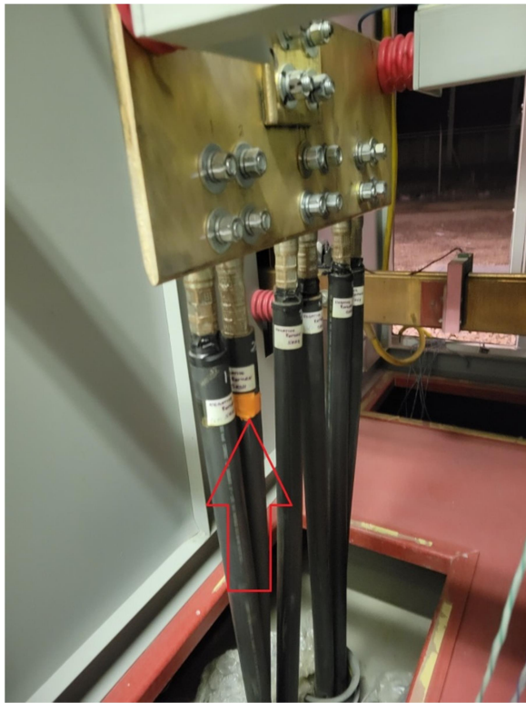
Feeder Cable #2 (counted front to rear) tested 2.6MOhms
