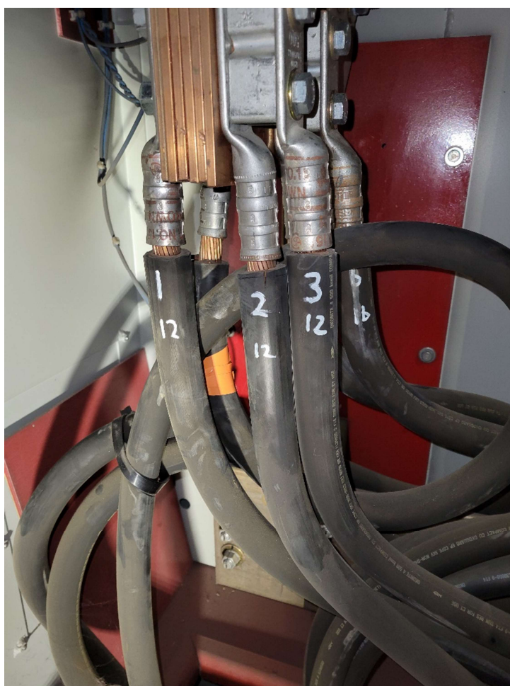
Failed POS cable marked with orange tape inside Feeder Breaker 2
