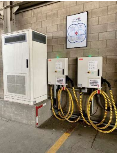
Plug-in charging infrastructure
