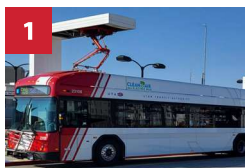
Meadowbrook Bus Charging Infrastructure
