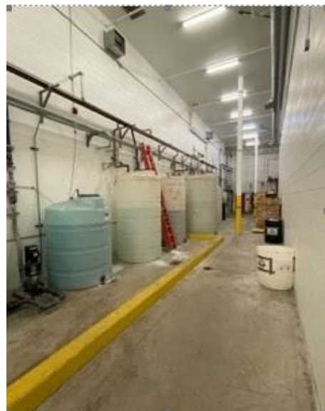
Figure 2 - Jordan River Service Center Mechanical Room
