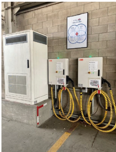
Plug-in charging infrastructure
